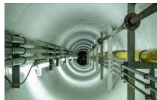
Low pressure pipelines
