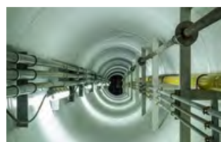
Low pressure pipelines
